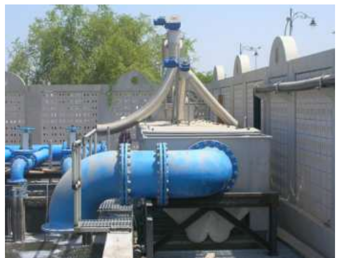
→ Compact grit and grease removal station
