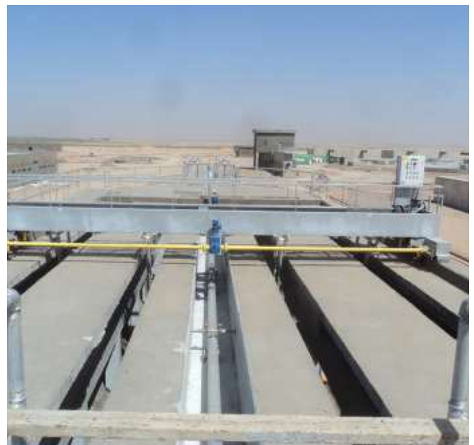
➔ Overview of the plant with degritting and degreasing scraper bridge for rectangular basin
