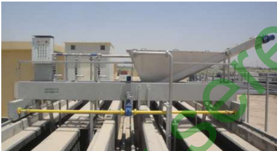
→ Overview of the plant with screw grit classifier
