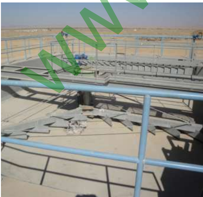
➔ Overview of the plant with grit removal unit
