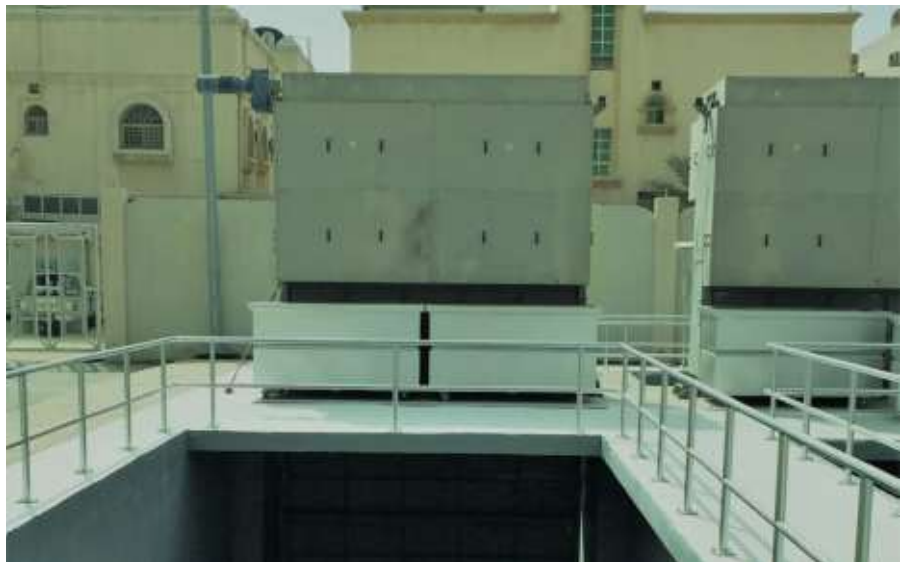
➔ Overview with GGPSC flat screens installed
