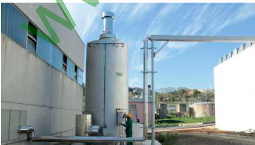
→ Filter for odour treatment biotrickling type
