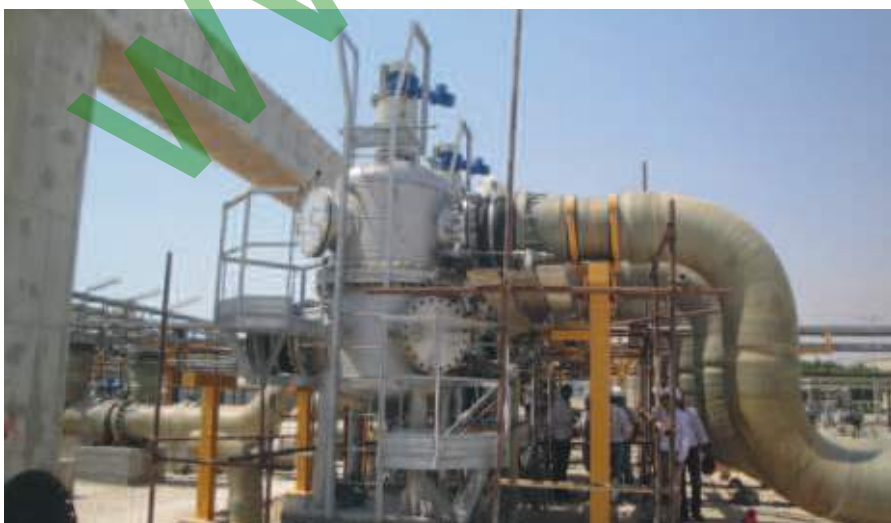
➔ Overview of the plant with automatic backwash water filter
