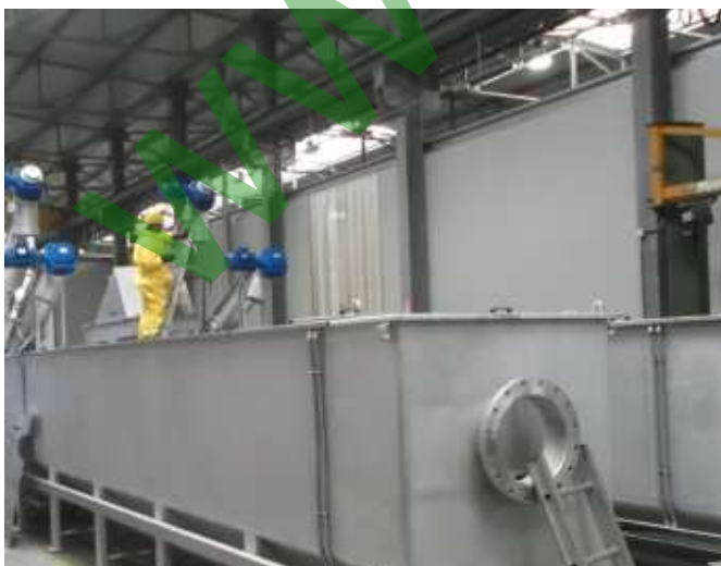
→ Compact grit and grease removal station
