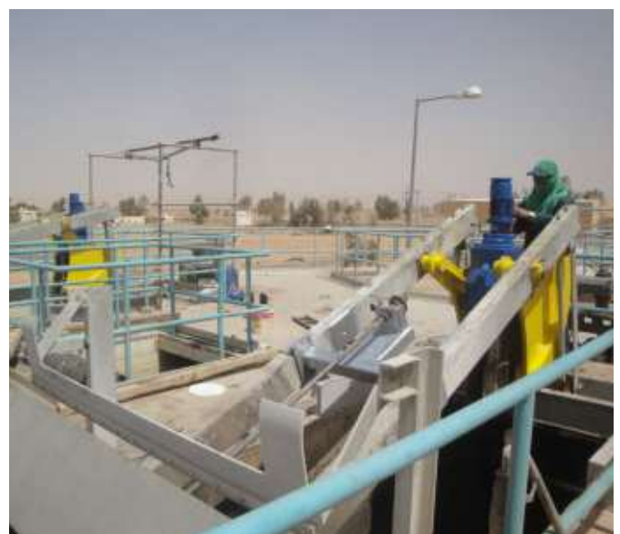
➔ Overview with GCMR type screens installed
