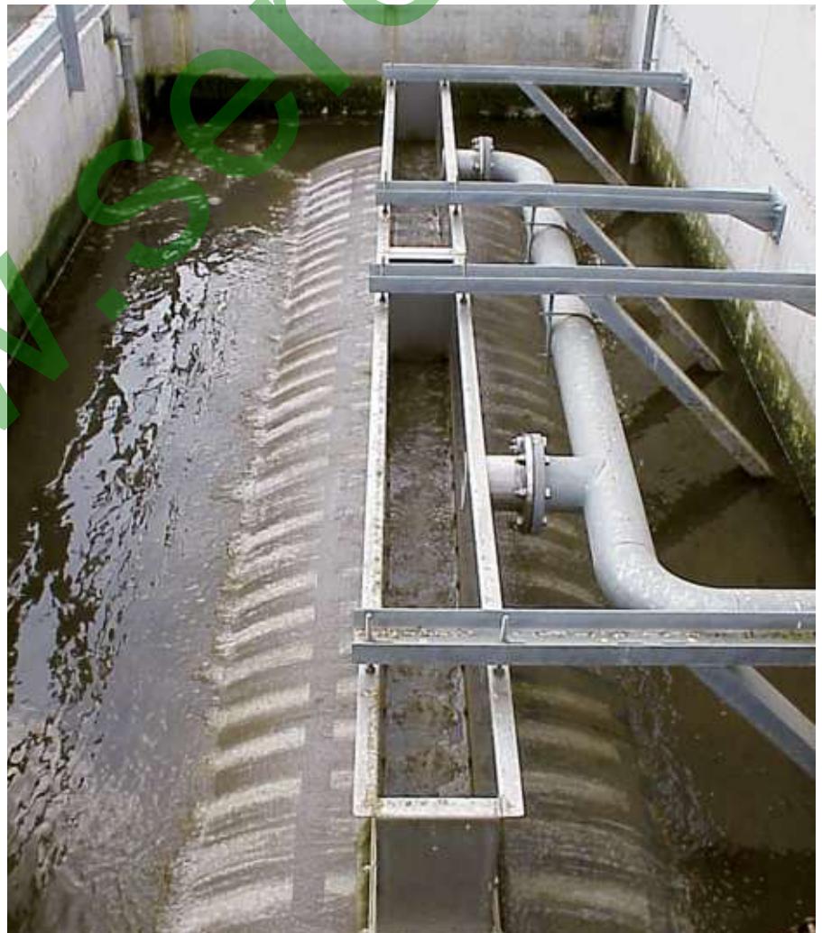
➔ Overview of the plant with gravity drum filter
