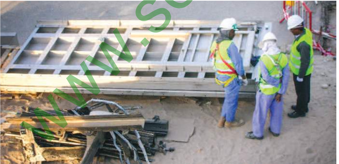
SERECO penstocks. PV4 model, installed at Sulaibya WWTP in Kuwait
