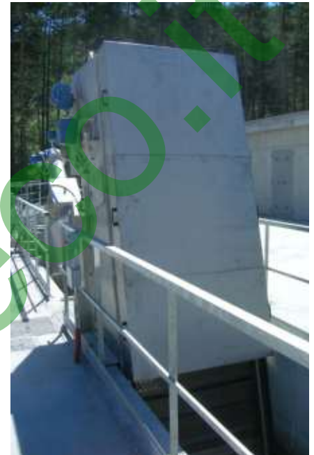
→ Belt screen GNAFO in operation
