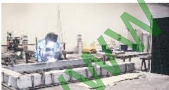
SERECO skilled welders at work with some penstocks to be installed in a wastewater treatment plant.
