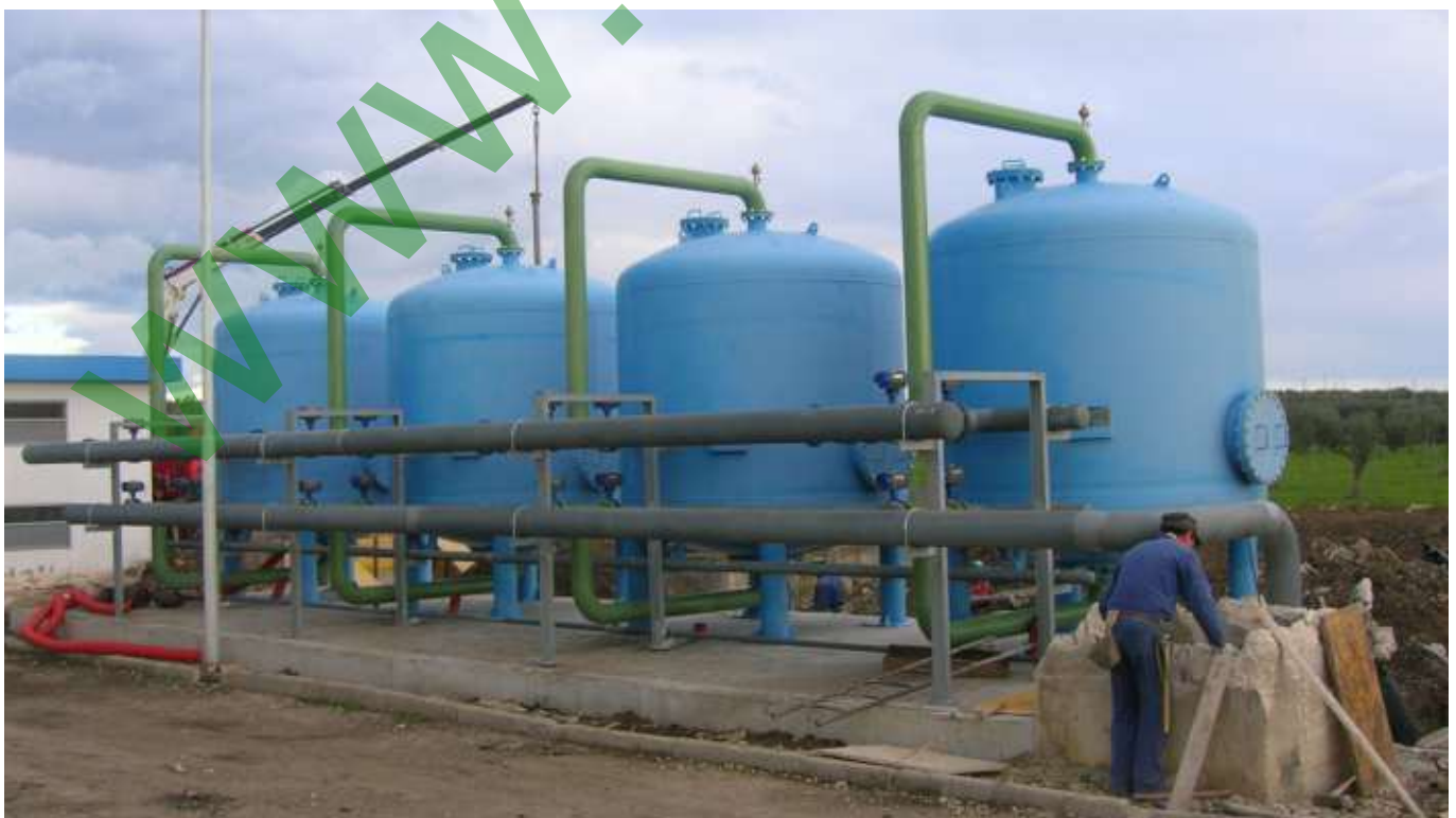
→ Overview of the plant with quartz sand water filter
