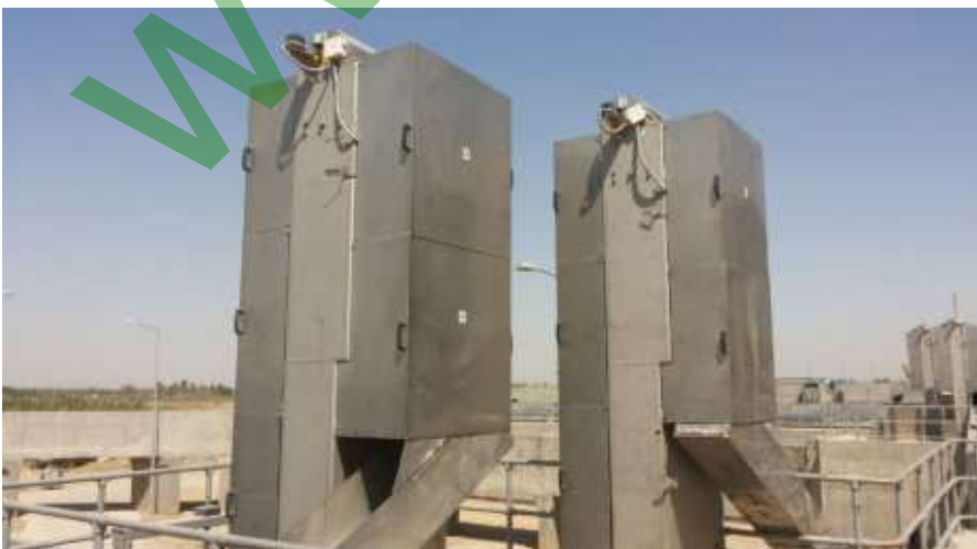
→ Overview with GPSC cable vertical flat screen
