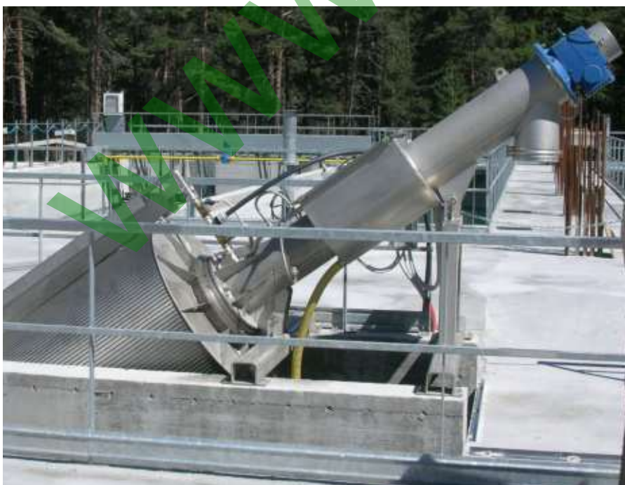
→ Installed FSSM screw filter
