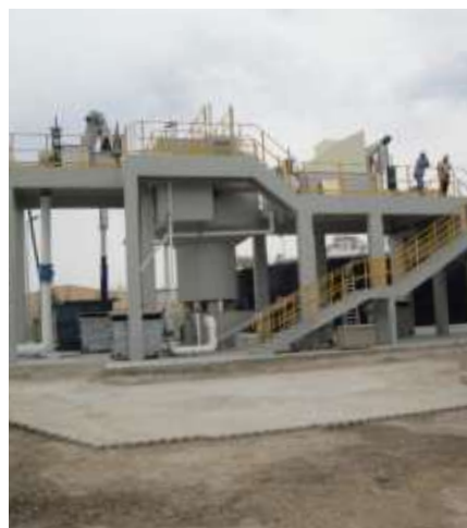
→ Overview of the plant with rotating blade sand remover with oil and grease separator
