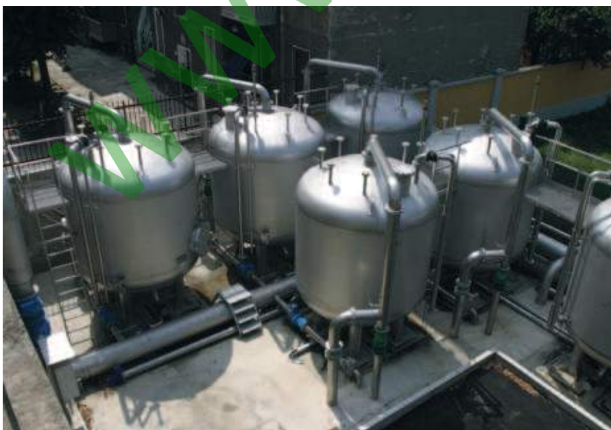
➔ Overview of the plant with activated carbon water filter
