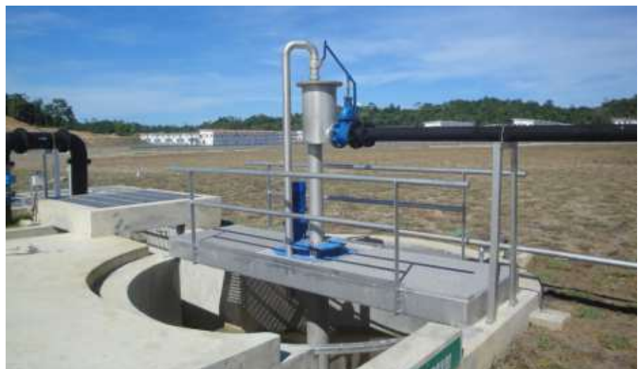
→ Overview of the plant with rotating blade grit remover
