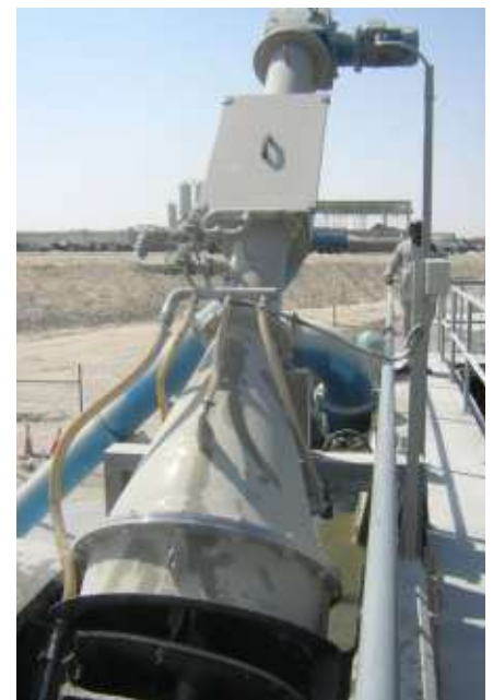
→ Screw filter FC installed
