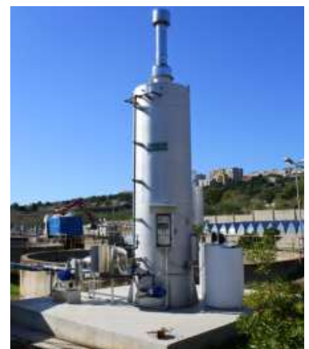
→ Filter for odour treatment biotrickling type
